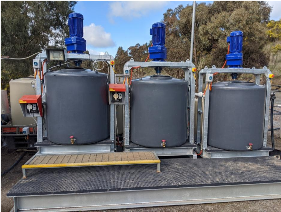
Figure 23 – Upgraded bioreactor plant
